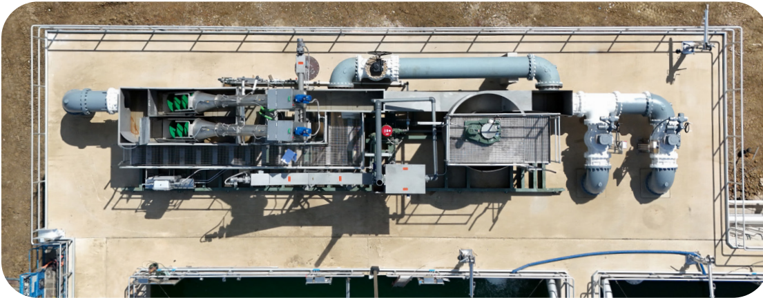
4.0 MGD PISTA®WORKS™ with dual fine screens and Model 15 grit screw conveyor with grit chamber bypass.
