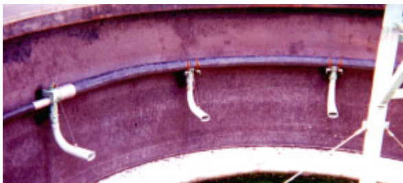
The Kraus-Fall design featuring the submerged inlet header can utilize either concrete or steel tankage.
