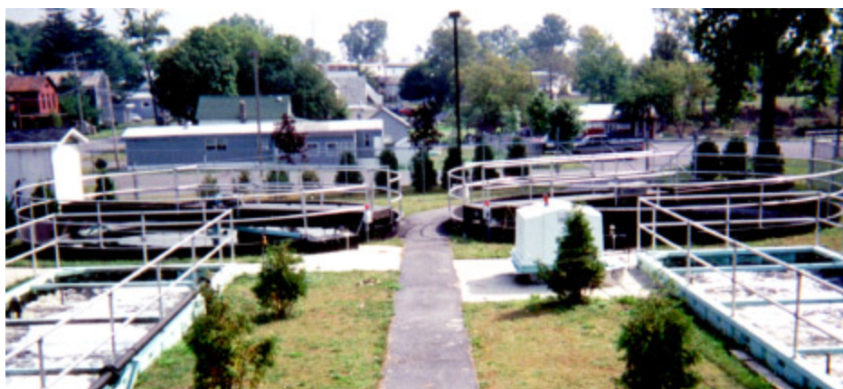
Applications for the Kraus-Fall Clarifier include final or secondary clarification and nitrification.
